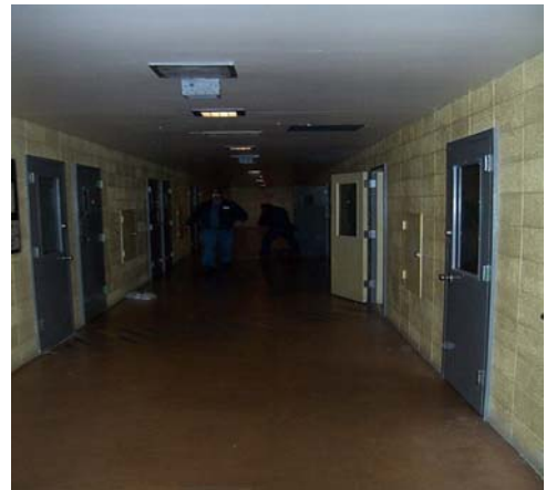
Juvenile Hall - before new lights installed
